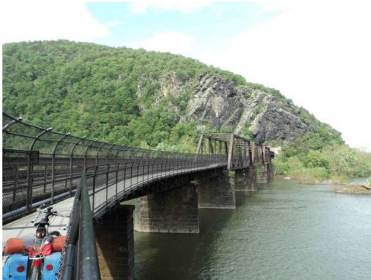
On the pedestrian side of a steel railroad bridge crossing the Potomac River from Harpers Ferry, WV back to the C&O Canal towpath in MD.
